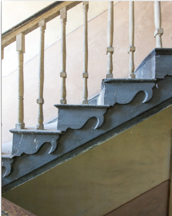
Figure 4 - Detailed joinery on stairway of No.4 Patrick Street Limerick – A Protected Structure
